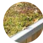
Additional Options for Flat Roofs Only Any variety of green roof, felt, EPDM or fibreglass
